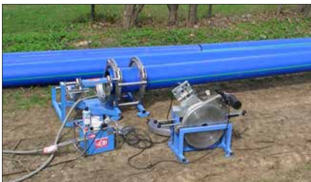
5.30 Gerodur service: provision of project-specific clamps for butt fusion (Widos) – delivery in robust heavy-duty box
