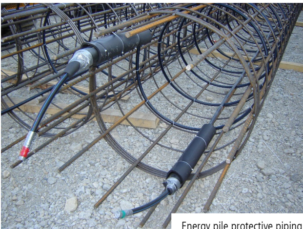
Energy pile protective piping
